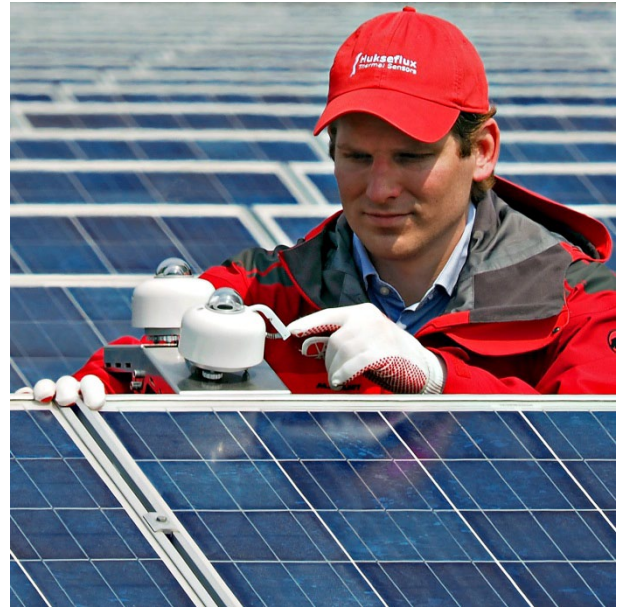
Figure 7 SR30 secondary standard pyranometers with digital output for GHI (global horizontal irradiance) and POA (plane of array) measurements
